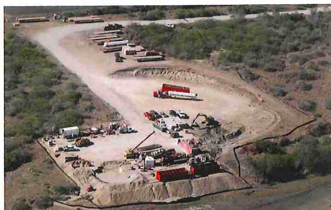
Laney's crossing of Nueces Bay in Corpus Christi, Texas, included two HDDs, one drilled from land on the north side and the other drilled from the port on the south side.
